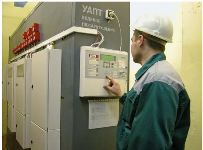
Servicing fire centre unit ESA
