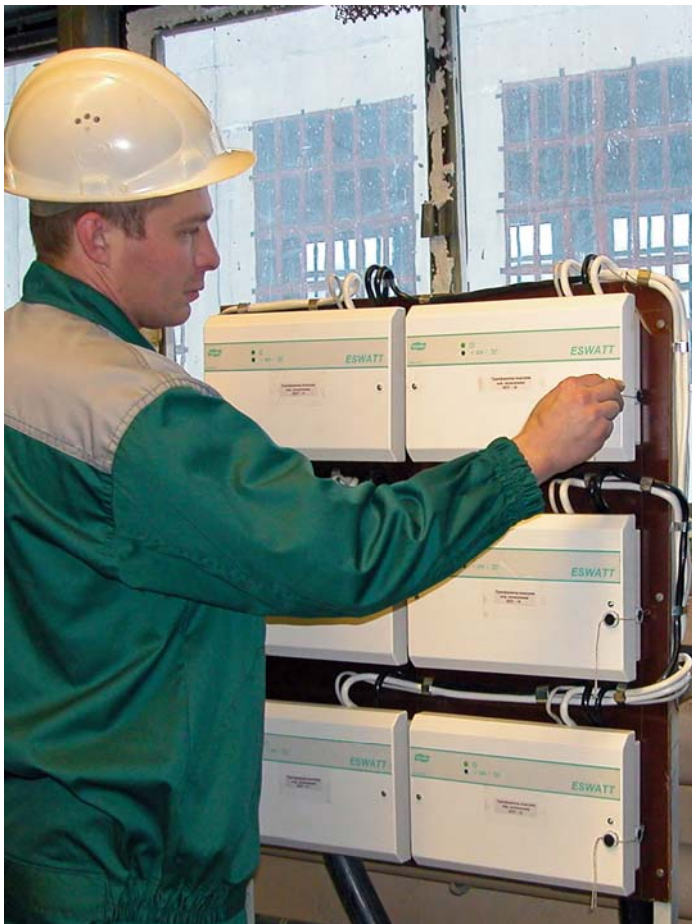
Checking operation of the Main Fire Centre, MESA
