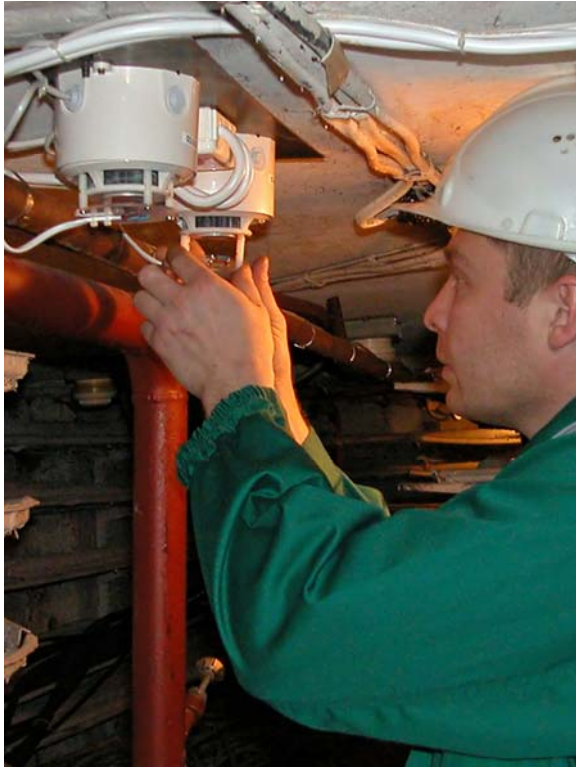
Servicing the fire detectors in situ
